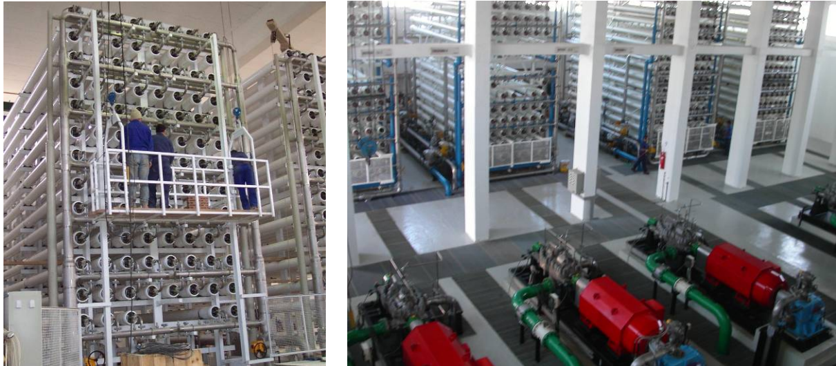
Figure 1-8: Left: Pressure cylinders containing the separation membranes of a reverse osmosis plant in Barcelona, Spain, with 30,000 m 3 /day desalting capacity; Right: RO-stacks and high pressure pumps of a 30,000 m 3 /day desalination plant in Gran Canaria, Canary Islands. Source: Mertes, DME
