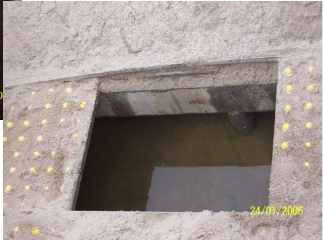
Sand Filter Problems
