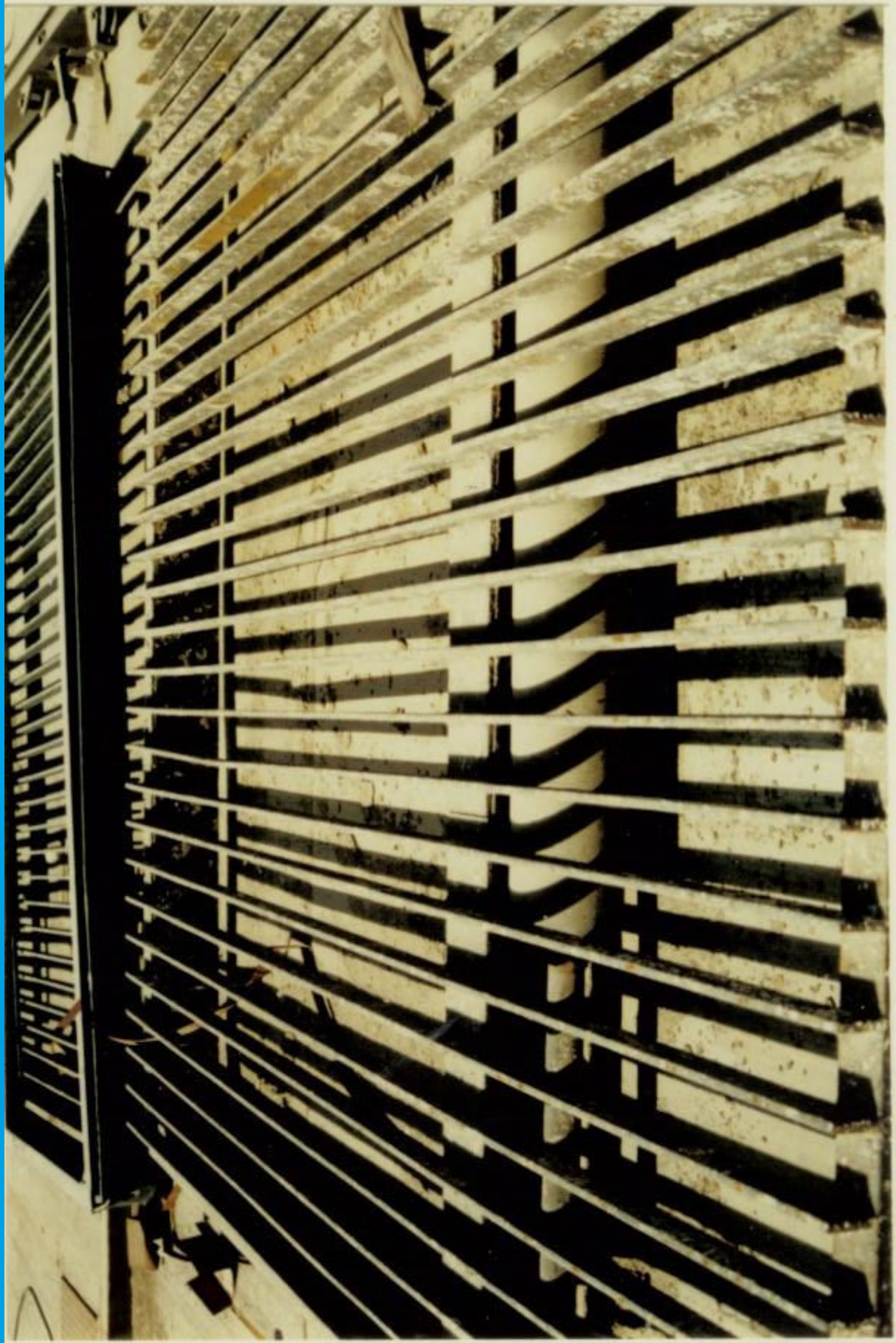
Screen bar 10cm wide at entrance of forebay
