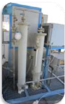
Activated carbon column
