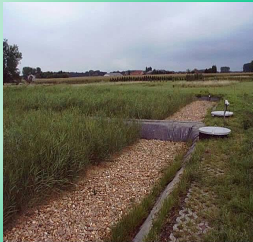
Sub-surface flow reed bed in Zemst, Belgium (Aquafin) , two beds in parallel.
