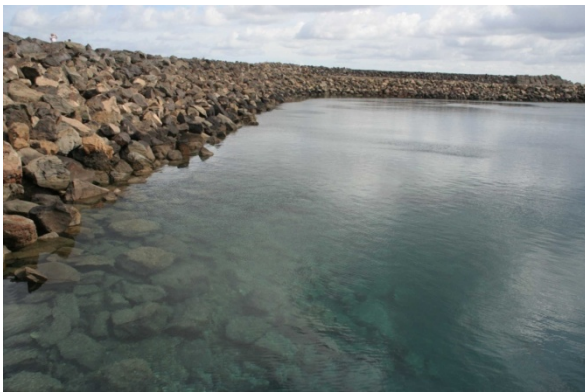
Figure 5: Open intake basin with breakwater.
