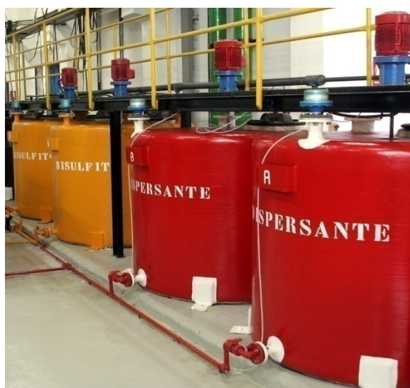
Figure 15: Pretreatment chemicals (top) and pretreatment dosing system (below).
