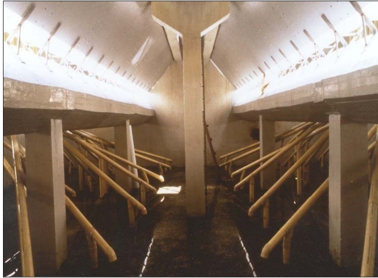
Internal view 1200 m 3 UASB, Cali, Colombia
